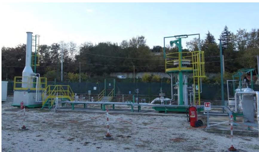
Figure 17-4 Rapagnano gas processing facilities (Source CGG)
