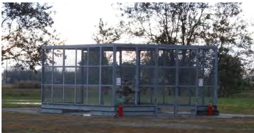
Figure 17-3 Sant' Alberto wellhead (source CGG)
