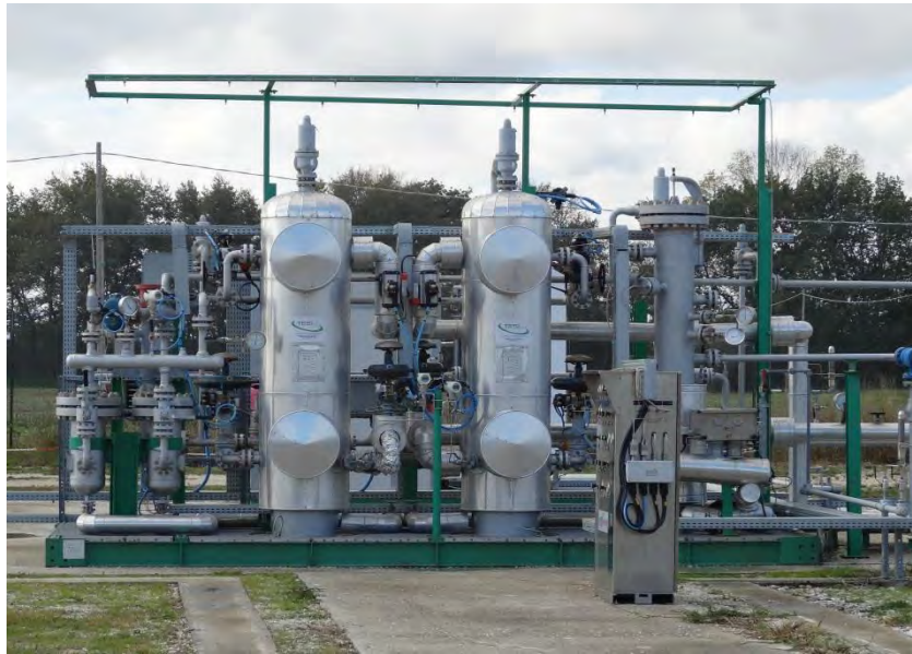
Figure 17-7 Casa Tiberi gas processing facilities (source CGG)
